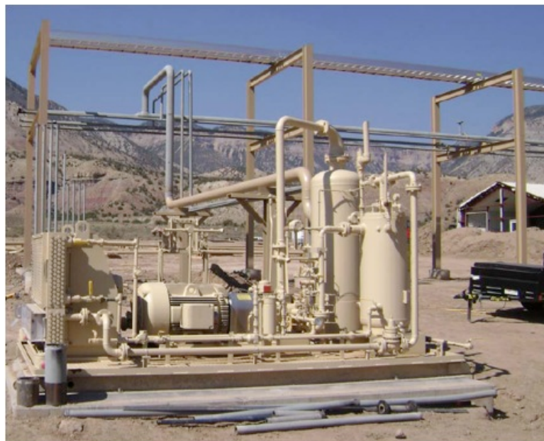
Vapor Recovery Unit in use by Williams.
